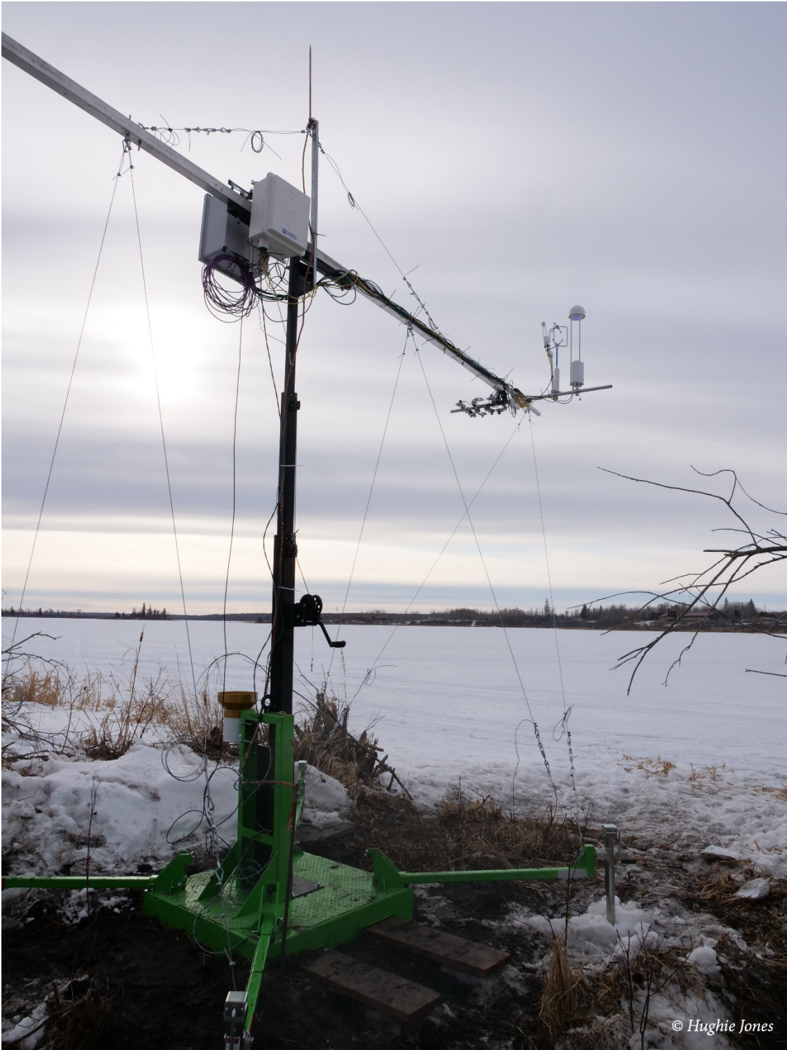
Fig. 14. Example of climate station supported by a telescoping tower.
